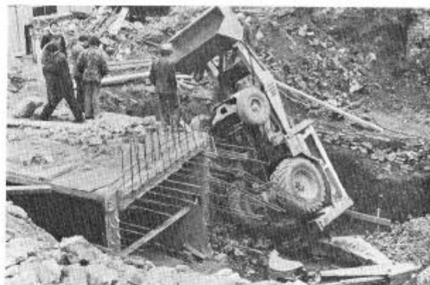
Fig 2: Collapsed J.C.B. in Area 2. (Photo: John Maloney)
