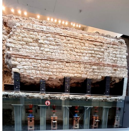
Above: interior face of the Roman city wall supported by underpinning jacks.
