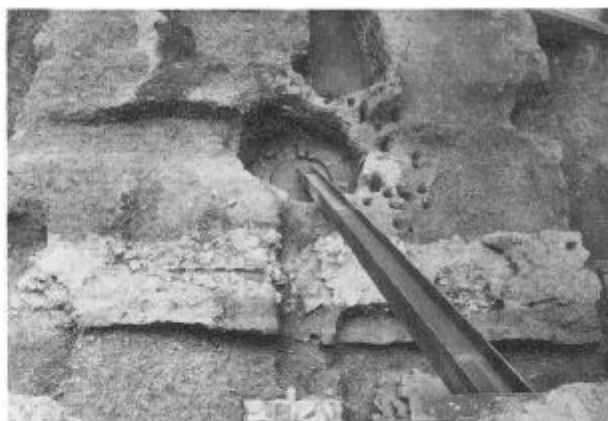
Fig. 4: Building A: looking east over the possible Roman road onto part of the west wall, corridor and burnt internal surface.
