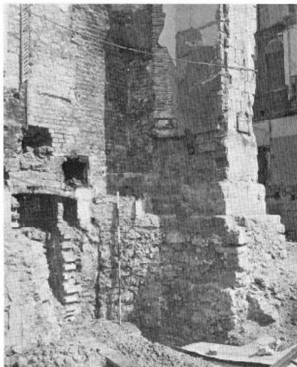
Fig. 8: A straight joint separating the foundation of the south-west corner tower from the west crypt wall. (Photo: P. Marsden)
